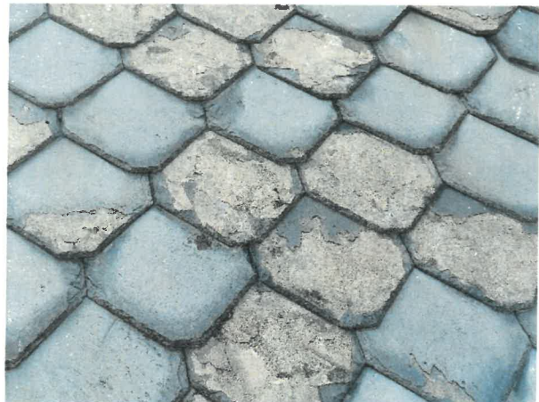
Photo 10: Deteriorated slate example 1
