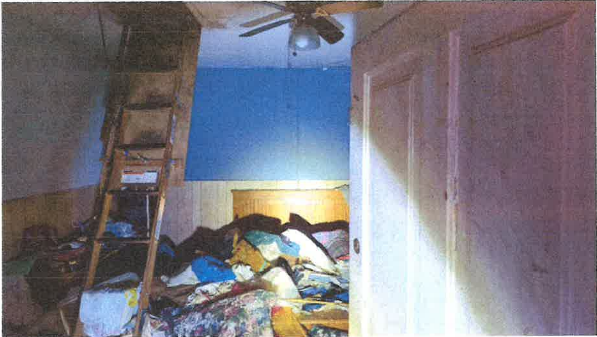
Photo 9. This is the upstairs bedroom with attic access. The floor in this room was also damage by water and was no longer safe.
