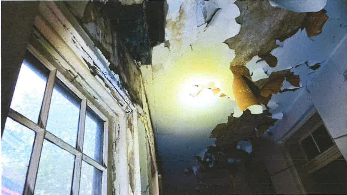
Photo 7. This is the north hallway on the lower floor. It was a former porch. There was extensive water damage to the exterior walls, ceiling and floor.
