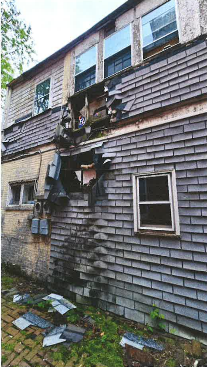
Photo 4. This is the remaining north side of 111 Hanover Street. Note excessive damage to the frame walls.
