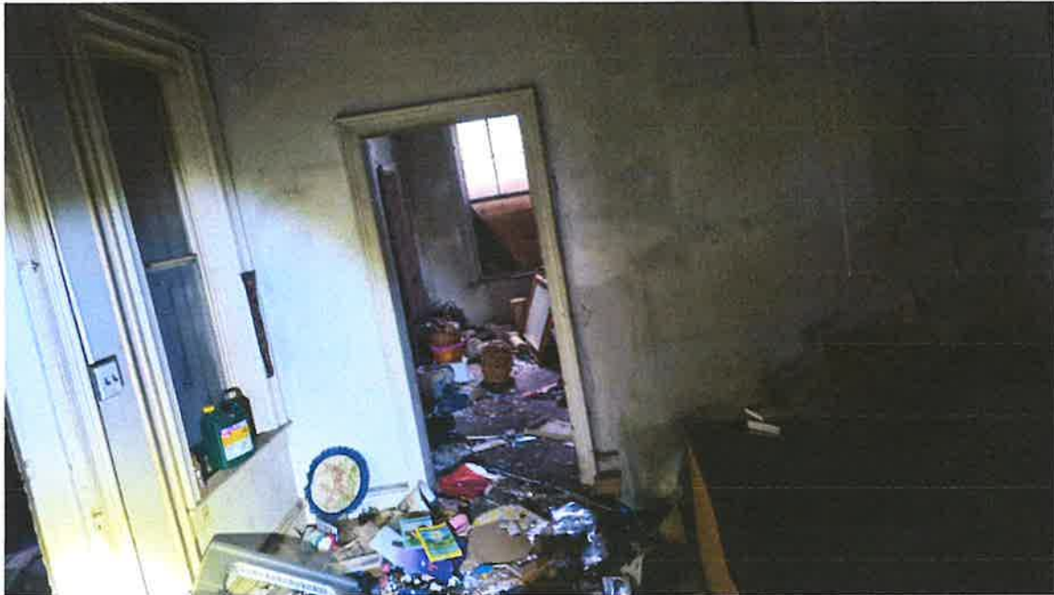
Photo 6. This is looking east on the first floor. The floor was unstable and not safe to walk on.
