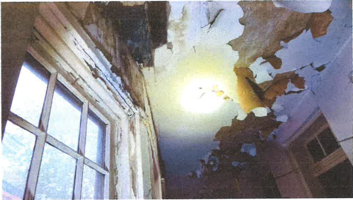
Photo 7. This is the north hallway on the lower floor. It was a former porch. There was extensive water damage to the exterior walls, ceiling and floor.
