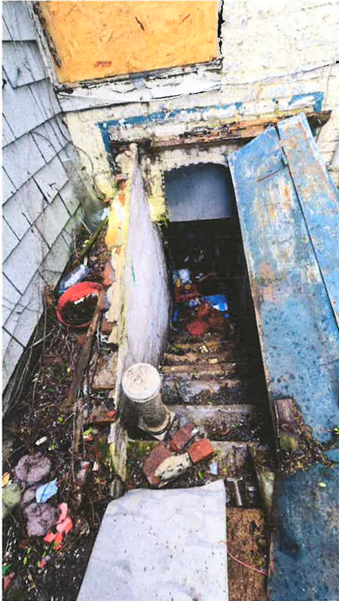
Photo 5. This is the basement entry on the east wall. There was too much debris to safely enter the basement.
