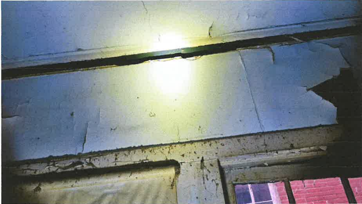
Photo 8. Separation of outside wall at enclosed porch. Wall has pulled away from ceiling by over an inch.
