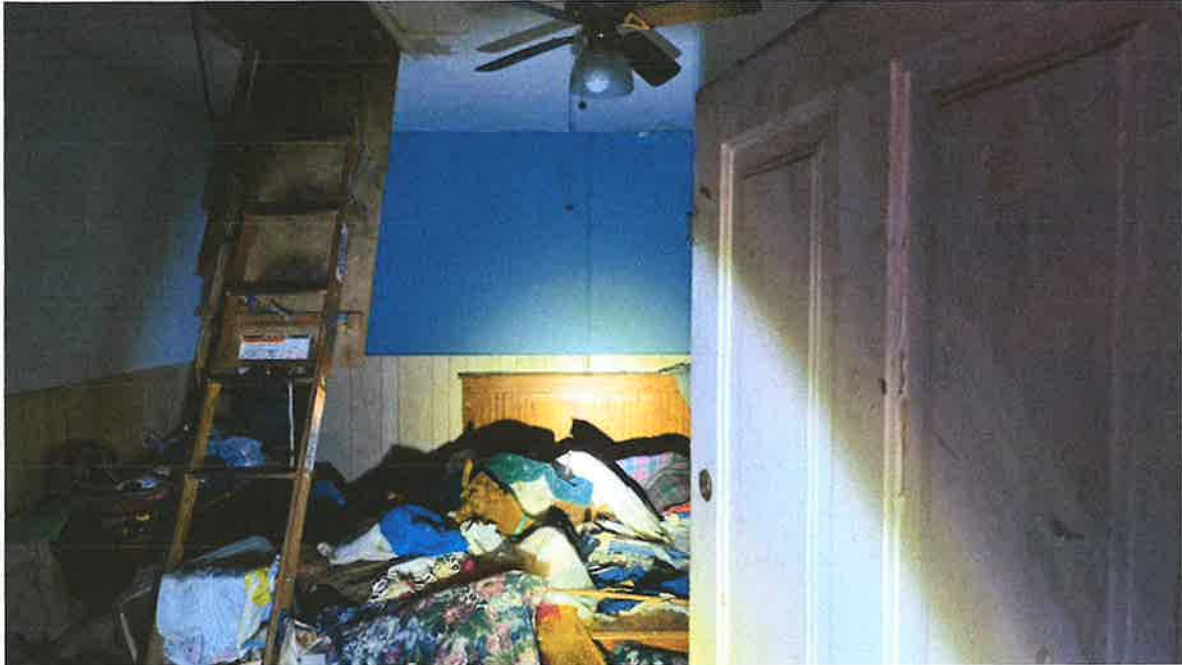
Photo 9. This is the upstairs bedroom with attic access. The floor in this room was also damage by water and was no longer safe.
